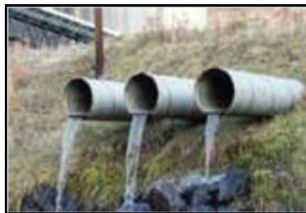
An outfall that is sending water into a storm drain or stream when there has been no rain in the last 72 hours.
